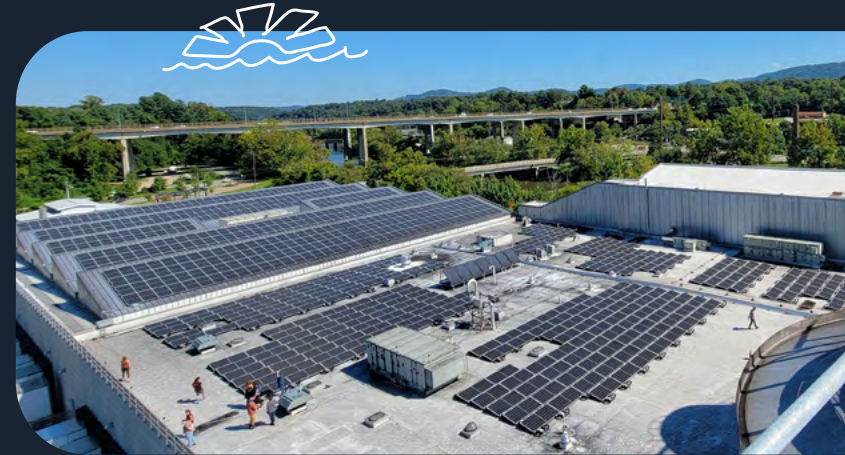
Solar array at Asheville brewery.
