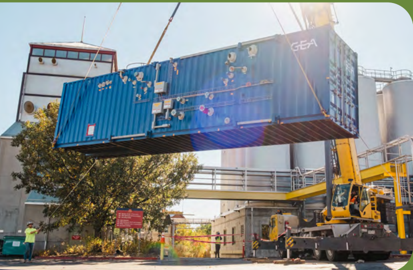
Installation of the core CO 2 recapture system at the Fort Collins brewery in fall 2024. The blue enclosure houses the primary equipment used to clean, purify, compress, dry, and liquefy fermentation CO 2 , preparing it for reuse throughout brewing and packaging operations.
