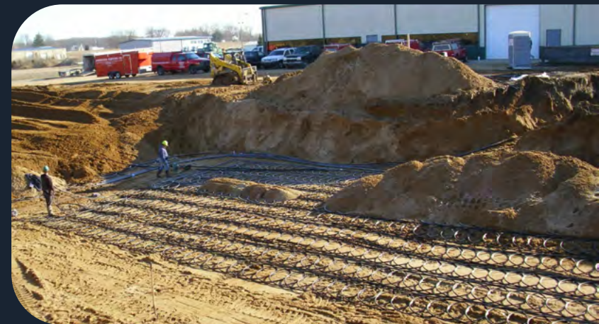
Geothermal system installed underneath the hop field at Bell's Brewery in Comstock, MI.
